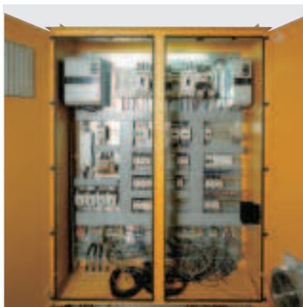
Figure 4: Example of a switching installation for the automation of machines and systems, each with a share of the power section and control section.
